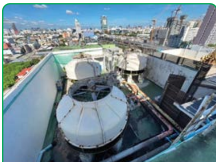
Existing air conditioning system
